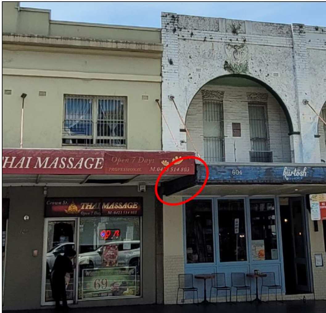
Figure 54: The existing interface between the awning of the neutral building (left) and awning of the contributory building (right)
